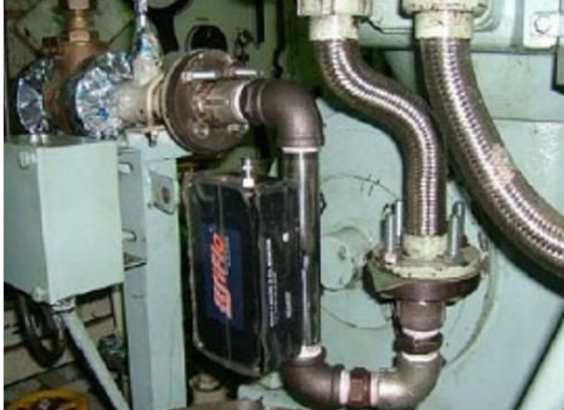
Typical installation in lubrication system.
