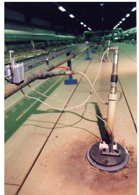
CellaTemp PS Pyrometer installed at the top of a tunnel kiln, including protective accessories
