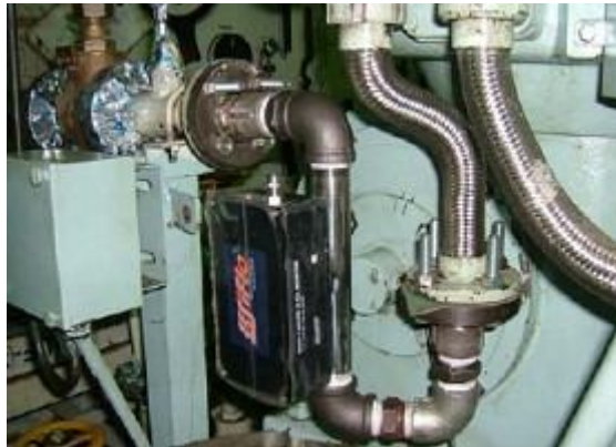
Fig 1.0 EESIFLO's water sensor installed On a ship purifier system
